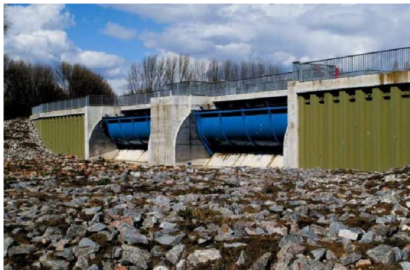
Figure 4: an example of an inlet construction as found in the German part of the Rhine River.
