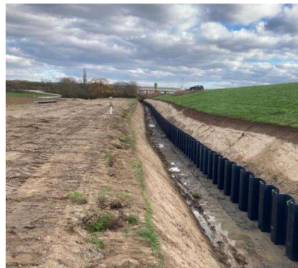
Figure 27. Trench for pile driving is not packed/dense.
