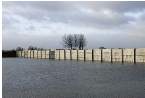
(b) Hondsbroeksche Pleij, located in the floodplain of the IJssel just downstream of the IJsselkop bifurcation. The picture shows the inundated floodplain and the structure almost fully. Photo: Rijkswaterstaat (2012)
