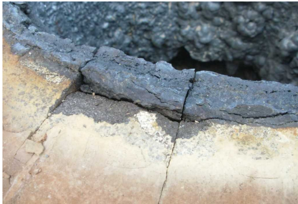
Fig. 1 Thermal crack in refractory mortars and bricks
